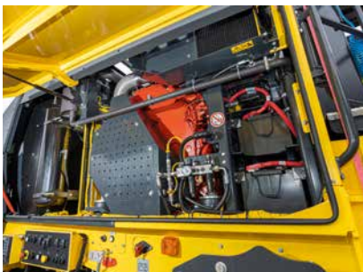
The batteries and compressed air system can also be easily accessed from the side.
