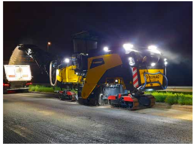
Full beam ahead: the BM/65 with Advanced Night Package on a motorway construction site.
